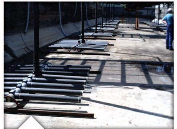
These liftable fine bubble tube grids on guide rails have worked over 10 years in this municipal WWTP
