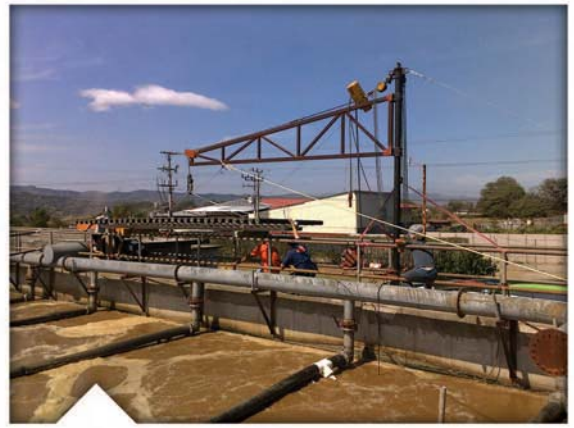
Retrievable grid with SSI Snappy Saddle™ Diffusers and a 304 SS frame replacing an underperforming floating lateral system
